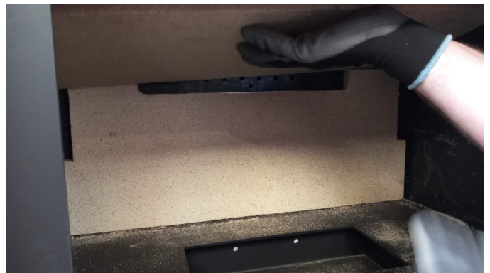
Position the baffles at the bottom of the combustion chamber and remove the upper baffle first and then the lower baffle.
